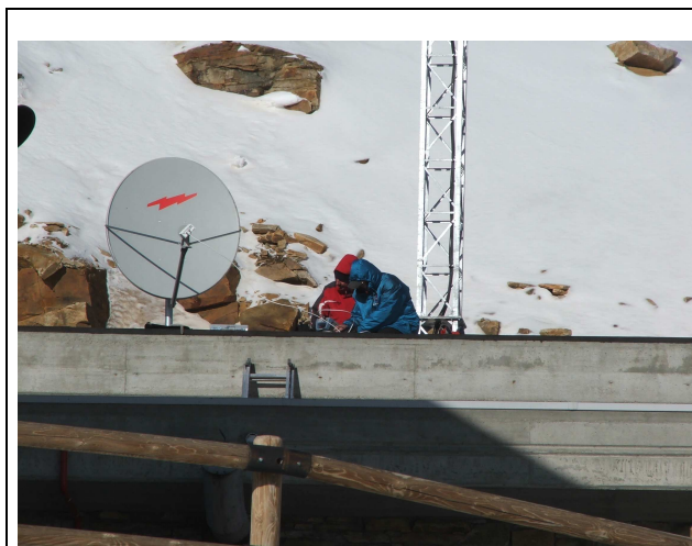
Station sismique SATI - Installation système de transmission
